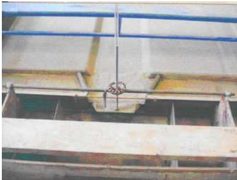
Figure 4.4 Tilting gate placed at the channel outlet.
